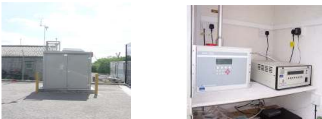
Figure 3 - Air Quality Monitoring Station Larne Harbour
